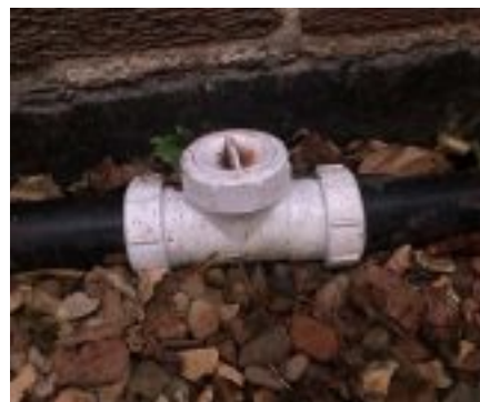
Non-return valve in pipework, to prevent backflow.
