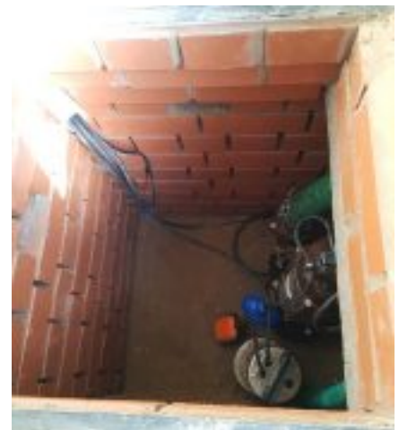
Two sump-pumps in lounge.
