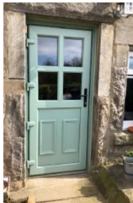
Flood door fitted.
