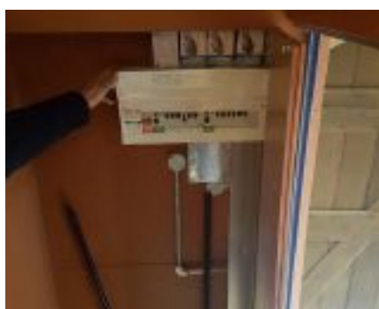
Raised electrics with drops from ceiling level.
