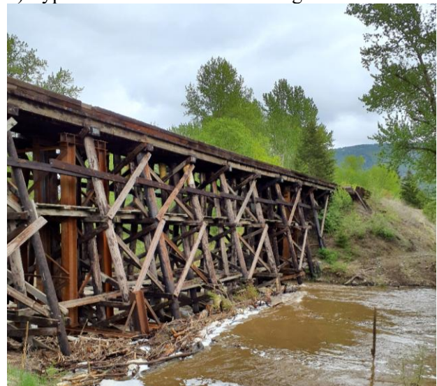
d) Wood trestle bridge accumulating debris.
