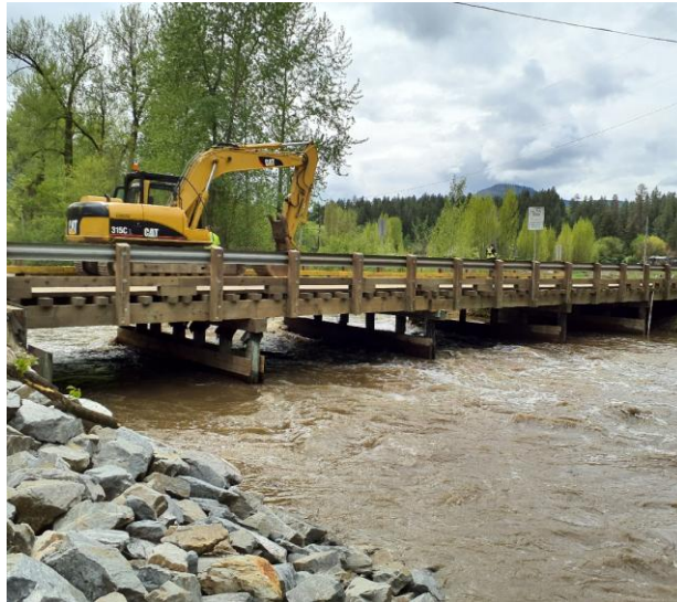
a) Multi-pier bridge with debris being removed
