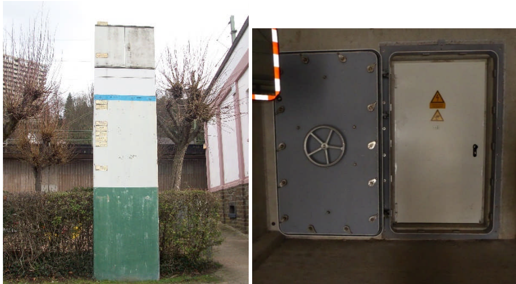
Figure 2: left: enlarged power substation (source: Gall 2015); right: power substation sealed with a submarine door (source: Gall 2015)
